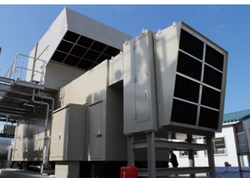
Power generation equipment at the Chiba Plant
